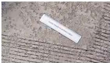
Figure 1: Typical scaling seen on concrete pavement
