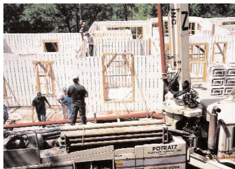
Insulating concrete form construction using concrete with 60 percent slag cement, 30 percent portland cement and 10 percent fly ash.
