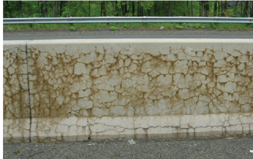
Fig. 1: ASR causes expansion and cracking of concrete structures and pavements
