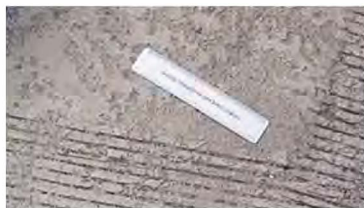
Figure 1: Typical scaling seen on concrete pavement
