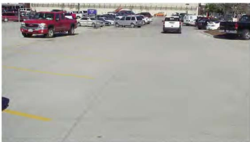
Figure 1: Typical scaling seen on concrete pavement
