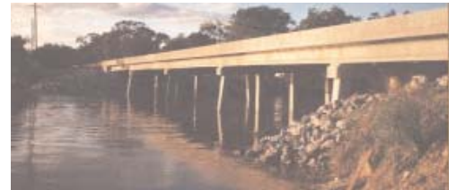
The Charenton Canal Bridge, Louisiana's first HPC bridge deck, achieved a chloride permeability of less than 2,000 coulombs, using a 50/50 percent portland-slag cement mixture.
