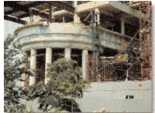
Figure 1: Greening occurred in concrete made with slag cement after forms were removed on the Canadian Chancery in Washington, D.C.
