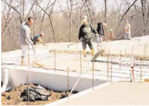
Self-consolidating concrete for residential floor slab using 50 percent slag cement, 50 percent portland cement.
